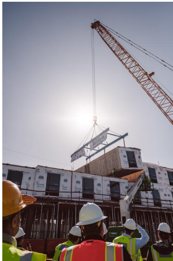
Constructing the Hilton Garden Inn San Jose (Calif.) Airport. Photo credit: Reggie Ballesteros Photography
