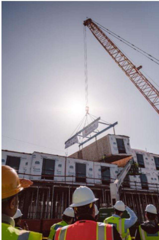
Stacking of the San Jose Hilton Garden Inn, a 150-room project A0 designed for developer Westlake Urban. (Photo courtesy of Reggie Ballestros)
