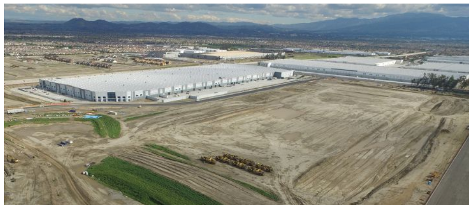
REDA plans to break ground on more than 4 million square feet of industrial real estate in the Inland Empire in 2021, alleviating some of the pent-up demand. One of those projects will be for ecommerce company Uline, which has experienced rapid growth since the pandemic.
